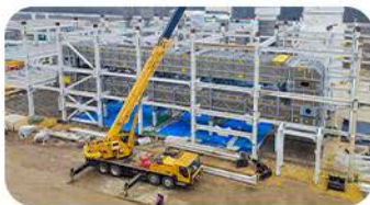
Solvent Extraction Capacity of 100-10,000 t/d
